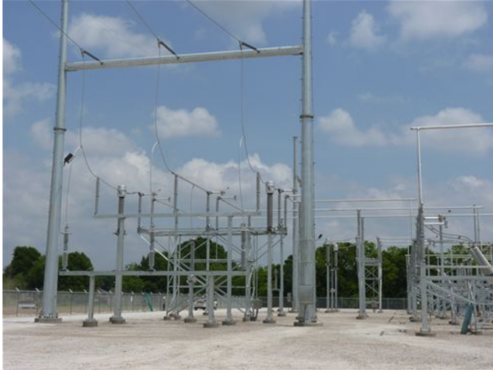
Figure 7: Termination Towers with H-Frames
